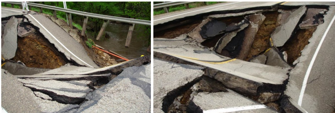
Figure 1.2.1-1—Roadway Collapse Due to Structural Failure of Culvert
