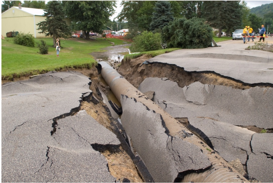
Figure 1.2-1—Roadway Collapse Due to Piping along Culvert and Loss of Backfill
