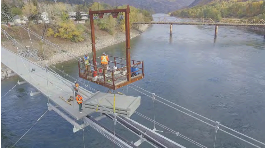
Figure C1.1-2—VIP-Molded FRP Panels Used on Suspension Pedestrian Bridge (Trail, British Columbia, Canada) (Source: Graham Group)
