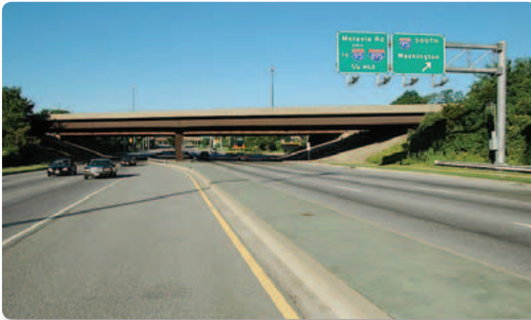
Figure 1-4 Simplicity and thinness are often enough. I-95 over Pulaski Highway, Baltimore, Maryland.
